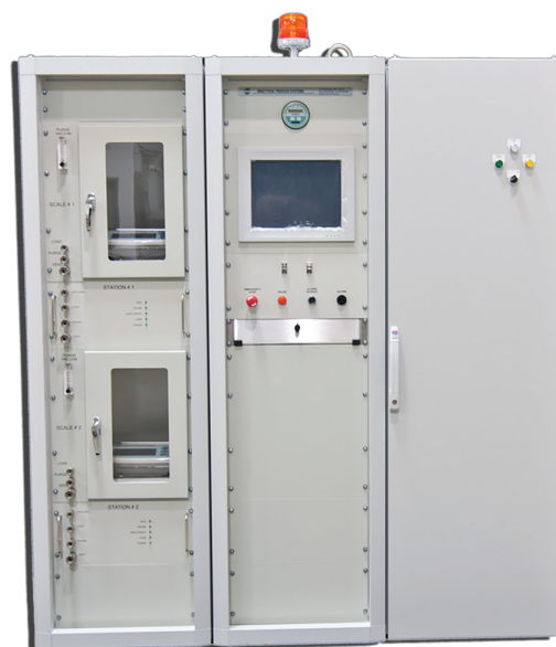
2 Station - 2 Scale system with Purge Air System attached
